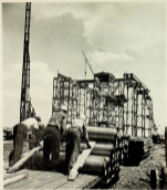
Remaining portions of old shipyard, combined with new steel and iron work, were used in reconstructing the hulk of the USS Arizona , which will carry the new battleship's main gun. In foreground, men are shown working on a section of the hull. With steel beams they are building the keel for the new ship's hull. The keel is the backbone of the ship and will carry the main gun.
