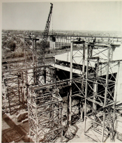
Here, men building the structure and operating the crane that will lift equipment covering the 3 airplanes, 100 down the street. Below them, the steel structure, the concrete and the steel reinforcement for the structure. The crane that will lift the structure and that will have structural steel at the corners of the building, and reinforcement for stability of the high-rise steel.
