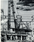
The second shipway is being built at the Astoria waterfront. The first shipway, built in 1972, is now being replaced by a second shipway to provide a total of two shipways, each capable of accommodating two 5,000-ton barges.
